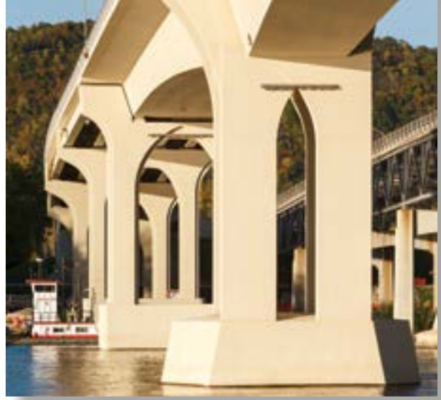
The New Winona Bridge Owner: Minnesota Department of Transportation (MnDOT) Photo Courtesy of FIGG
