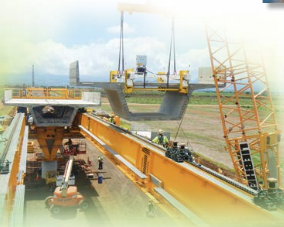
Owner: Honolulu Authority for Rapid Transit (HART) Honolulu Rapid Transit Viaduct Phase 1 & 2 Photo Courtesy of FIGG
